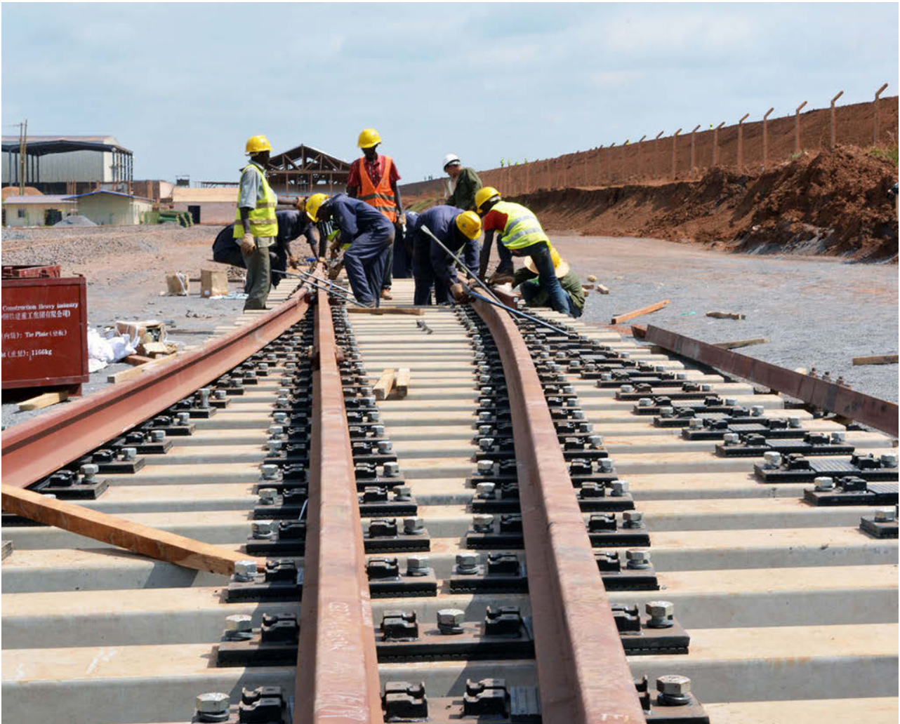
Construction of a brand new standard gauge railway (SGR) line from Mombasa to Nairobi. © Africa Business Magazine
