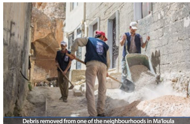
Debris removed from one of the neighbourhoods in Ma'loula
